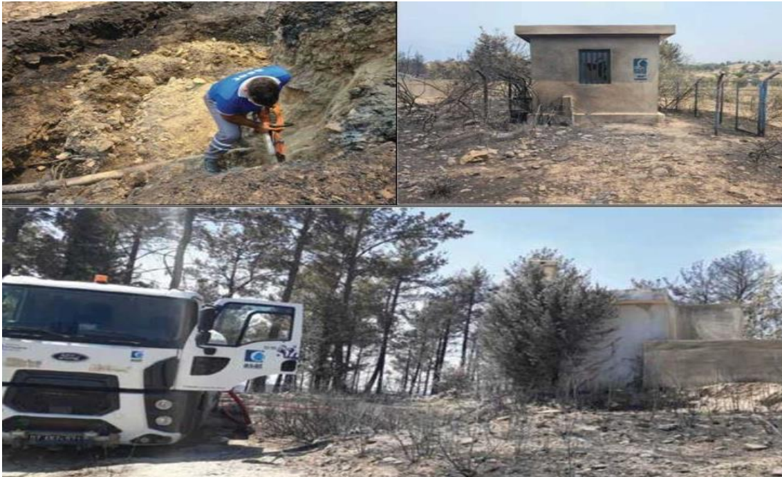
Figure 2: Situation of Affected Infrastructure After Wildfire Disaster (Images of Drinking Water Network, Water Storage Tank, Pumping Stations)
